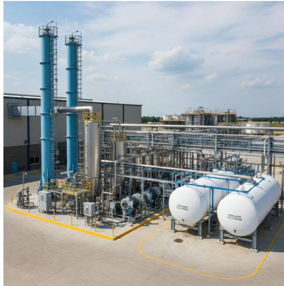
25 tons per day carbon dioxide recovery plant
